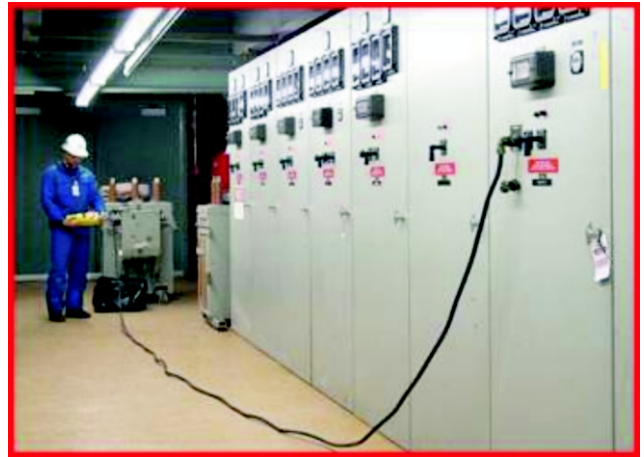
Fig. 5) Remote switchgear racking mechanism is an ENGINEERED to reduce risk.
