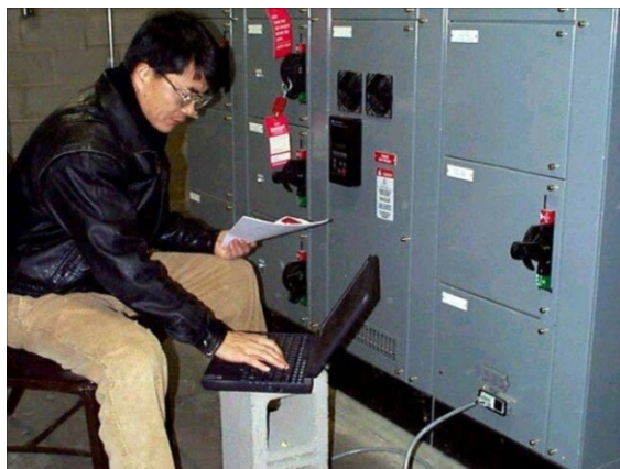
Fig. 4) Convenience Interfaces on Smart Motor Control Centers ELIMINATE exposure to voltage when troubleshooting.
